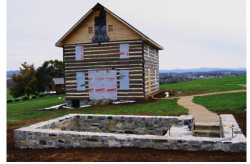
Pictured above are the recently constructed Weaver-Brunk Log House and the David Heatwole Cobbler Shop foundation to be completed in the near future.
