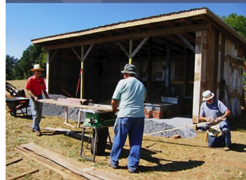
Cliff Lind, Larry Martin and Ervie Glick construct the Sugar Shack on September 10. It houses the hearth to boil molasses, a cider press and an old apple grader, all used during Harvest Day.
